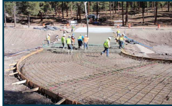
Location: Santa Clara, NM Client: Federal Highway Administration Project: Concrete Rigid Paving
